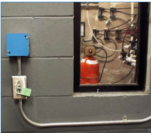
Chlorine gas room through viewing window
