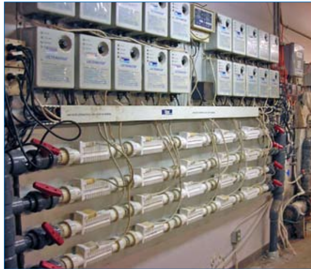
Electrolytic chlorine generators
