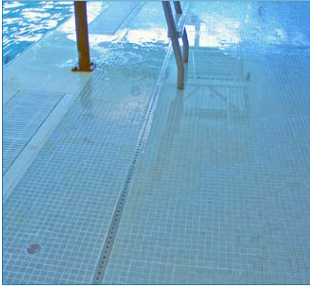
Example of standing water
